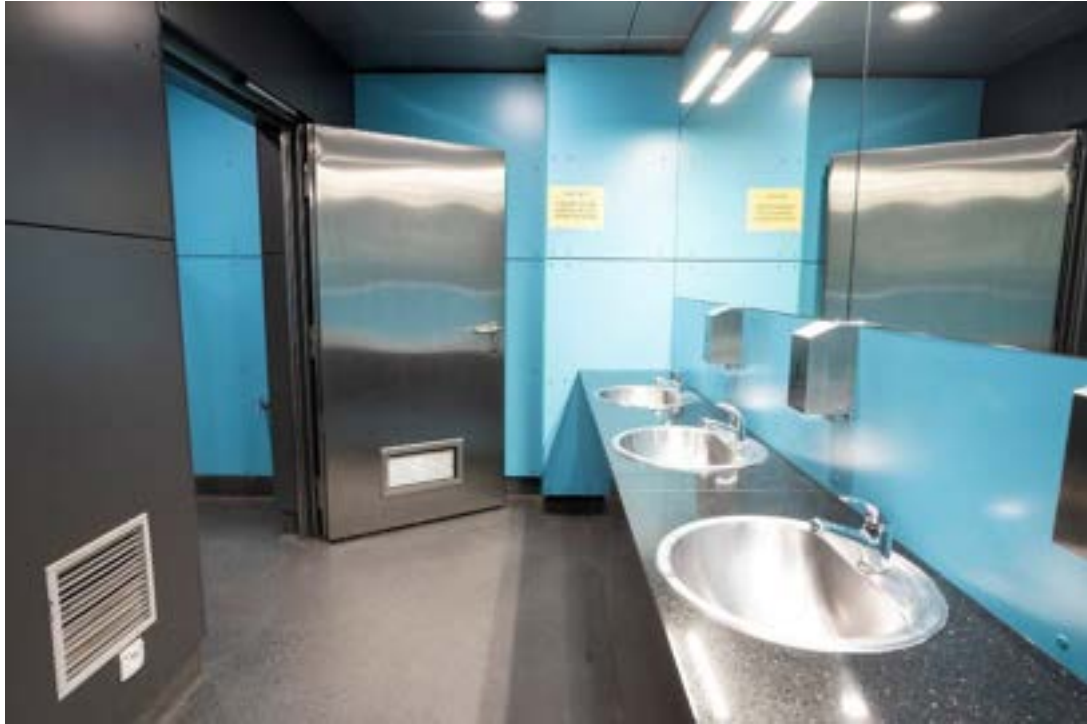
Fig. 3.6.4. Accessible and available toilet facilities in Warsaw metro. Color- and useful. Photo Credit: Metro Warszawskie
