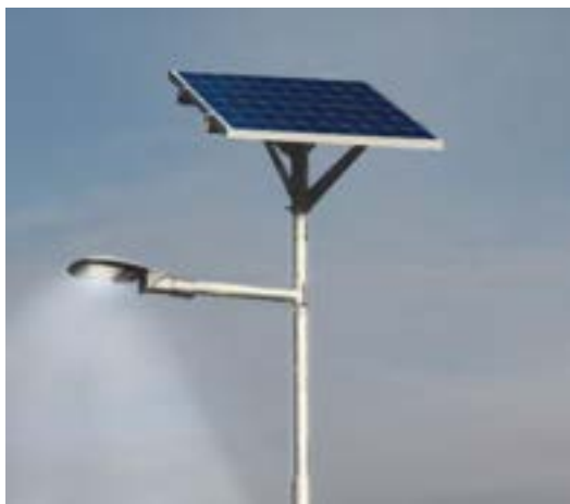
Fig. 4.15.2. Solar panel fuelled public lighting.
